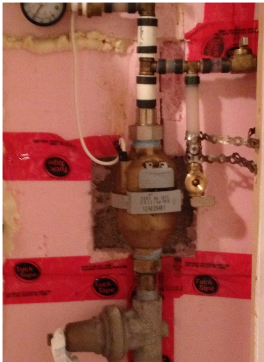
(c) Water Main Meter
