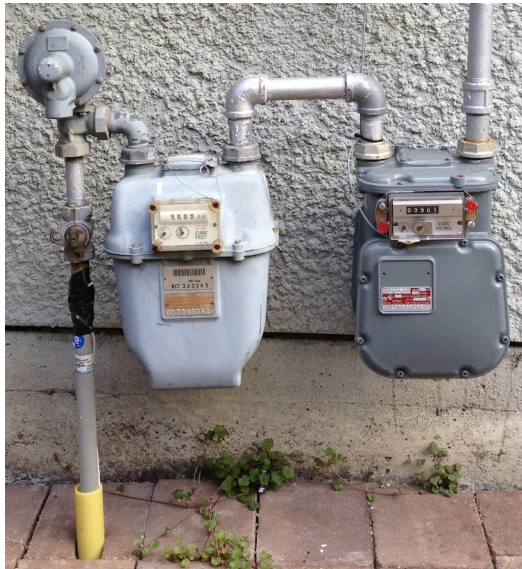
(a) Gas Main Meter
