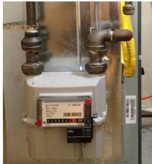
(b) Gas Furnace Meter
