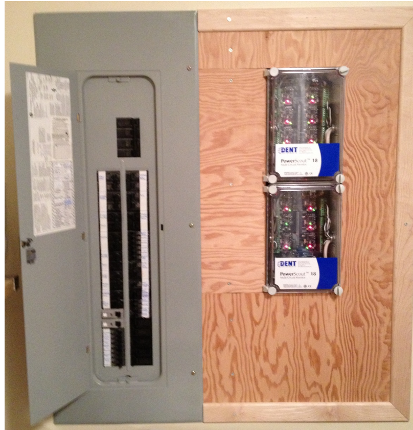
Figure 4.1: Two DENT PowerScout 18 units metering 24 loads at the electrical circuit breaker panel. Measurements are read over a RS-485/Modbus communication link by data acquisition equipment (see Figure 4.2(a)).
